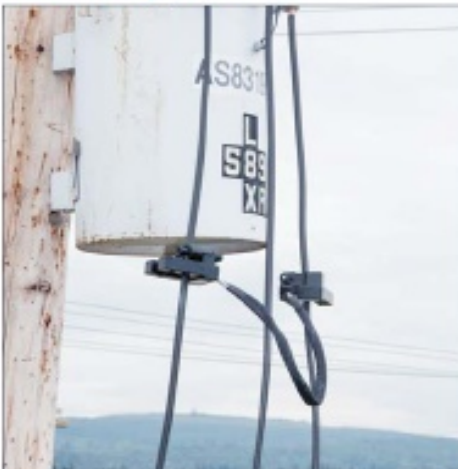
Overhead TMS deployment
